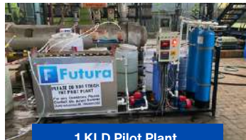
1 KLD Pilot Plant
