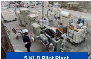
5 KLD Pilot Plant
